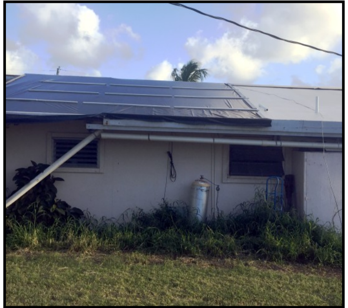
A large portion of the roof came off the building that house the WIVH studios
